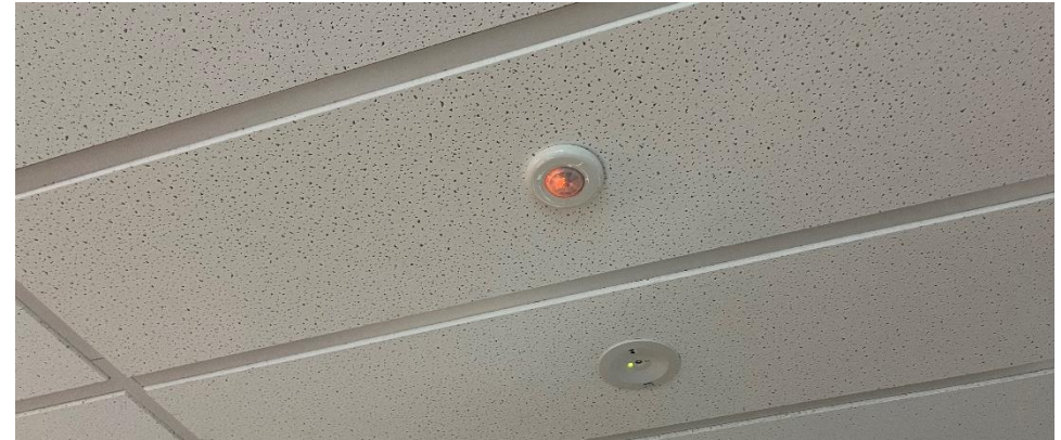
FIGURE 20: EXISTING OCCUPANCY SENSOR LOCATED ON THE CEILING.
