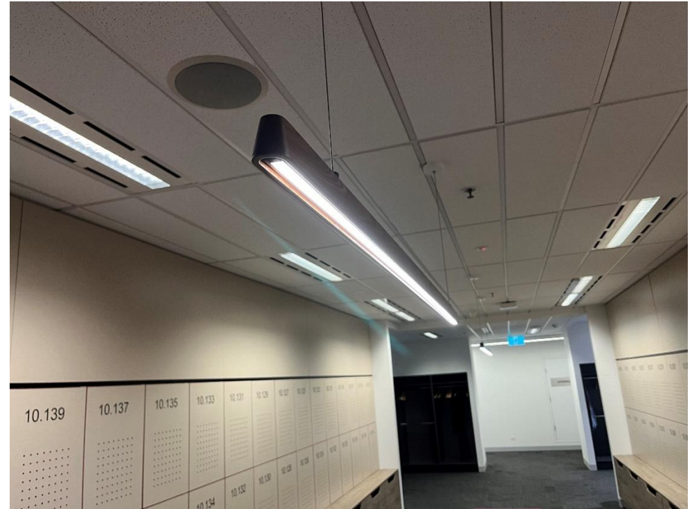
FIGURE 19: SUSPENDED LED LIGHT FITTING AND EXISTING RECESSED T5 FLUORESCENT FITTINGS (LOCATED ON LEVEL 10.)
