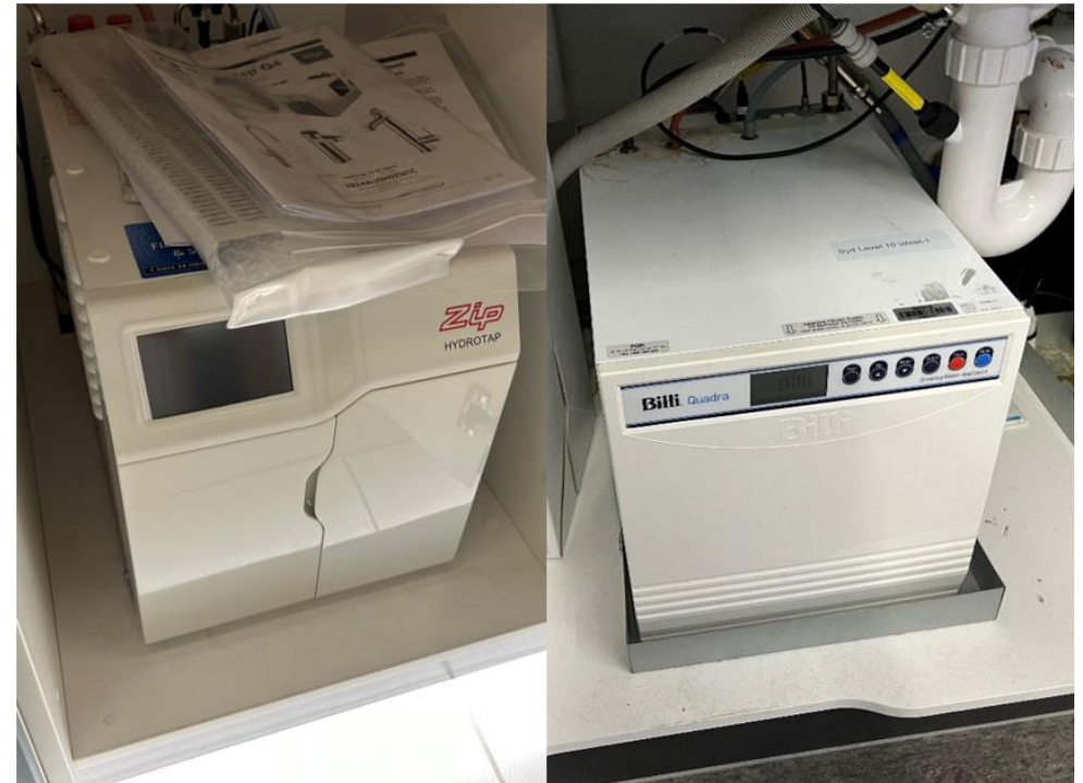
FIGURE 21: UNDER SINK ZIP HYDROTAP (LEFT) & BILLI (RIGHT) BOILING, CHILLED WATER UNITS
